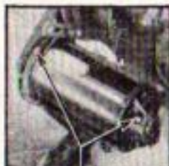
3000 MILES GENERATOR BEARINGS 2 POINTS USE ENGINE OIL
