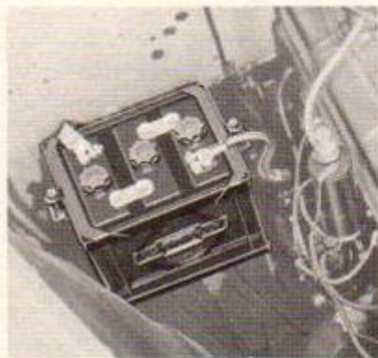
Fig. 31—Battery in Location
